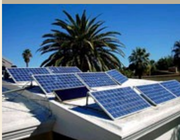
Solar Panels mounted on roof
